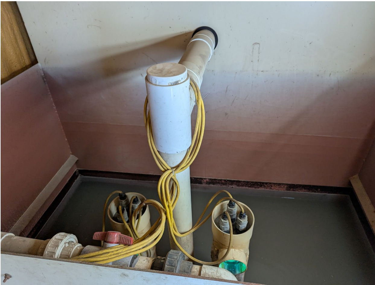
Figure 4. Inside the treatment plant where effluent sample is collected. UV lights inside white pipes attached to yellow wires.
