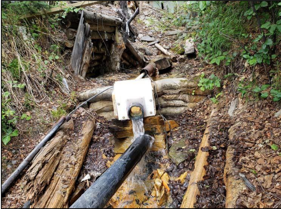
Photo 1. Onek adit discharging effluent with pipe disconnected.
